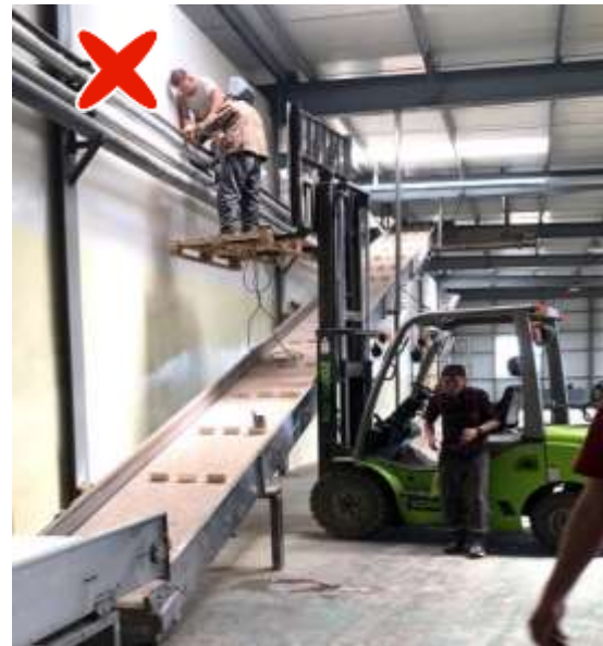
Figure 68: Badly prepared work at height using inadequate equipment with insufficient safety means
