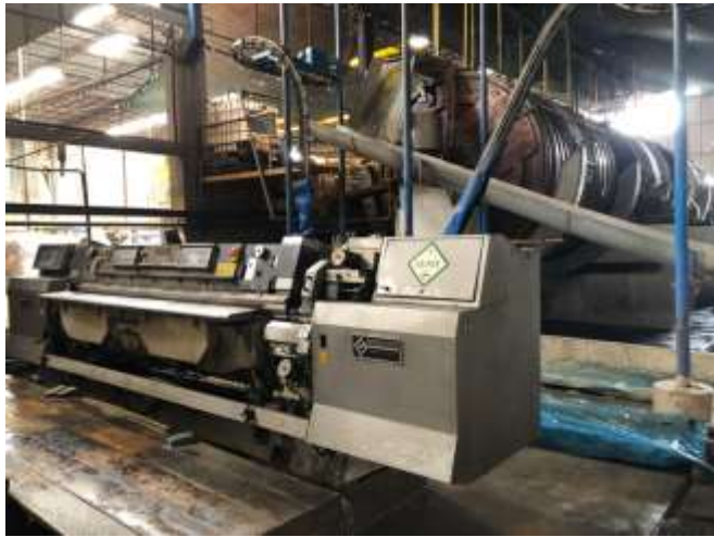
Figure 40: Well maintained beamhouse m/c improves safety and productivity
