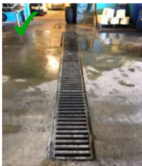
Figure 80: Cover floor openings and drains
