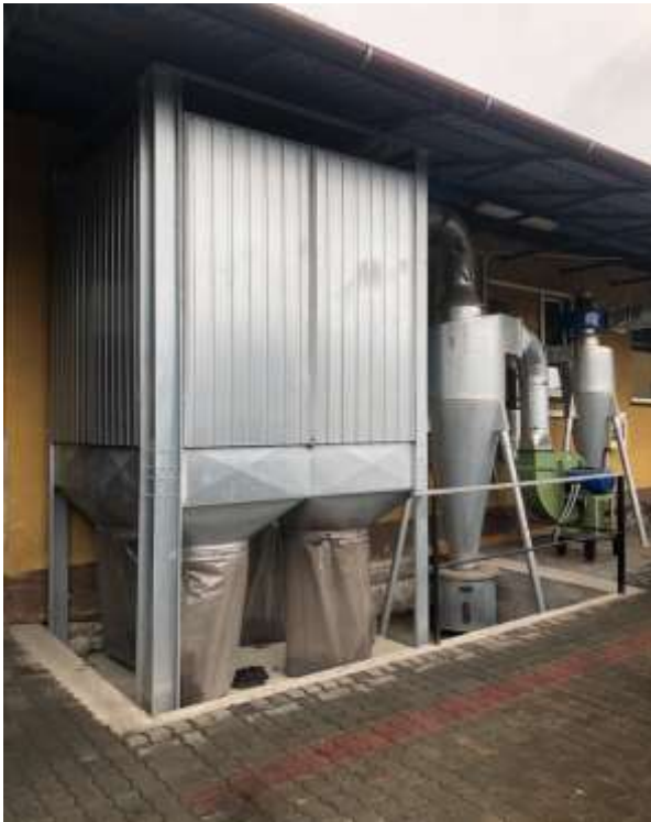
Figure 59: Outdoor part of the LEV. Dust extraction system cyclone + filter (air cleaner)
