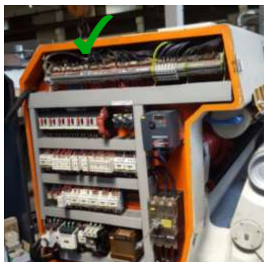
Figure 56: High safety standard of an electrical installation of a machine
