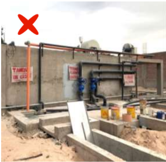
Figure 97: Open channels and confined spaces should be protected and access limited
