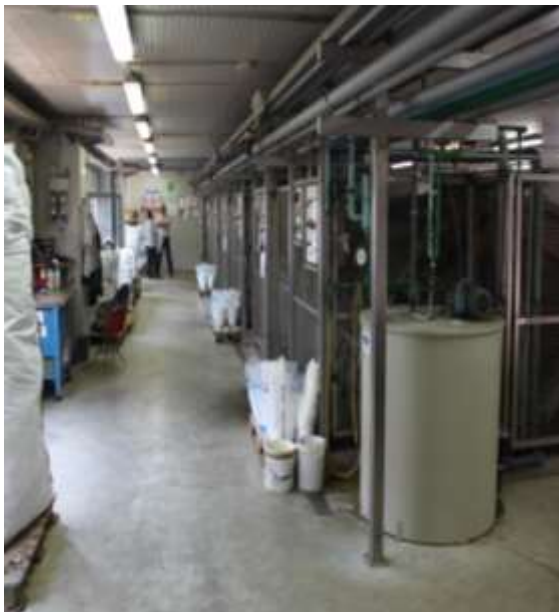
Figure 74: Good work organisation but no access routes nor chemical areas marked
