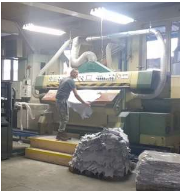
Figure 60: Indoor part of the LEV from the previous picture, installed on a shaving machine
