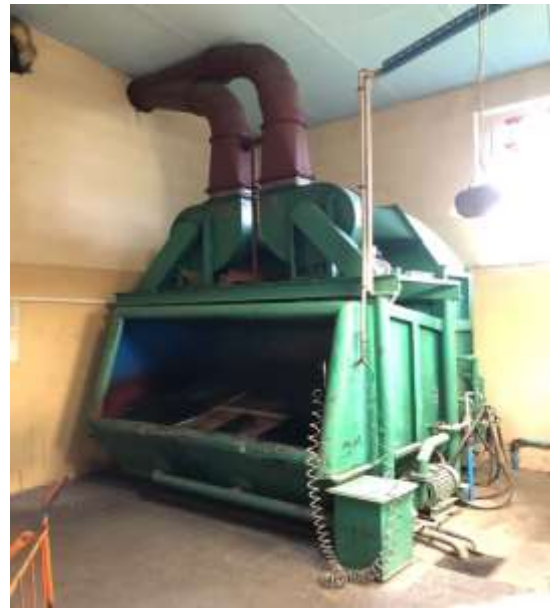
Figure 34: Spraying booth with and extraction system
