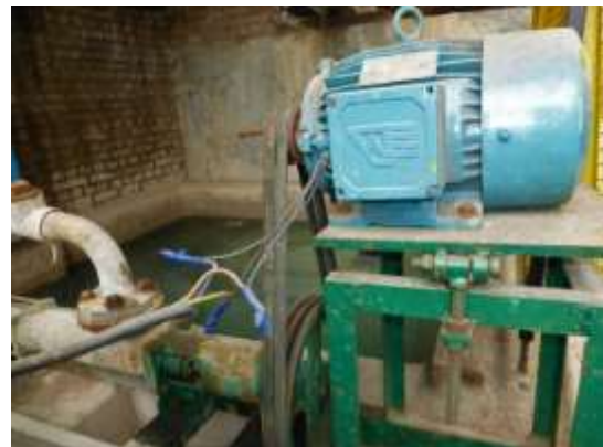
Figure 58: Don't allow open terminal boxes and missing cable glands
