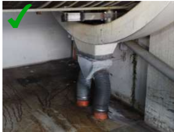
Figure 13: Modern "banana gutter" with a two-channel system allowing the separation of effluent
