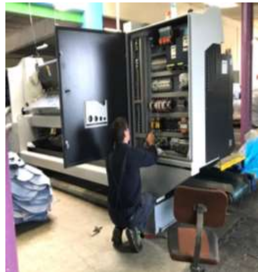
Figure 65: Regular maintenance and machinery review is crucial for safety
