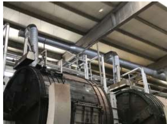
Figure 91: Air ventilation in beamhouse
