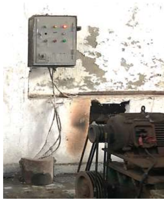
Figure 57: Check condition of electrical installations
