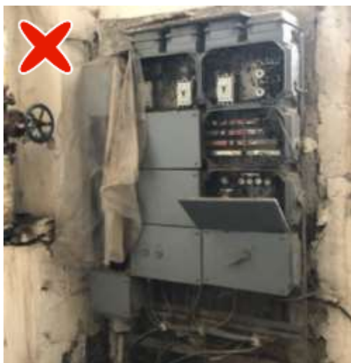
Figure 55: Poor safety standard of an electrical installation
